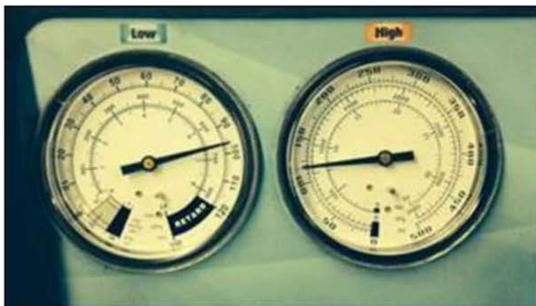
Figure 6. Equalized pressure condition. No pressure generated from compressor.
