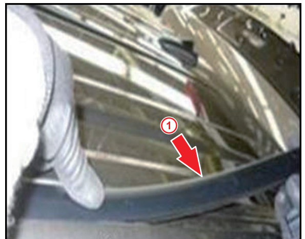
Figure 22. Incorrect Installation Technique
