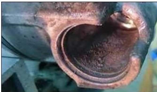
Figure 14. Corrosion in the N280 valve bore.
