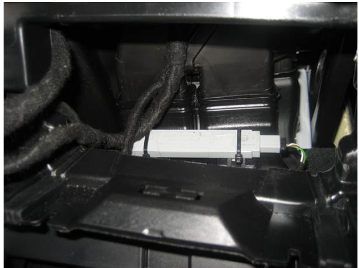
Figure 8. Aerial 1 mounted on HVAC ducting.
