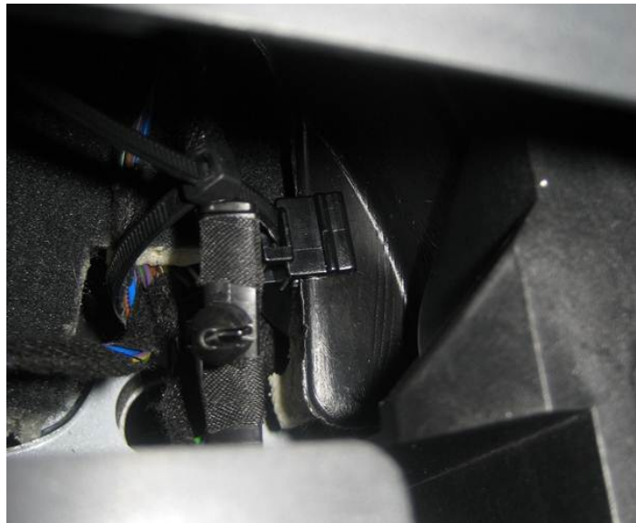
Figure 9. Zip tie needs tightening.
