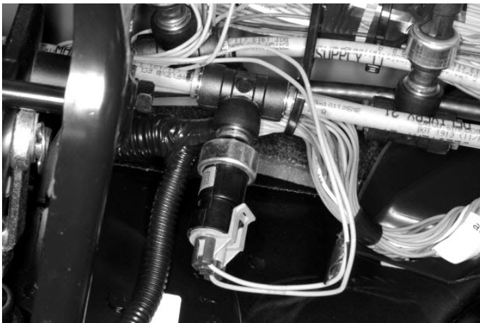
Figure 1 Pressure Switch: Original Installation
