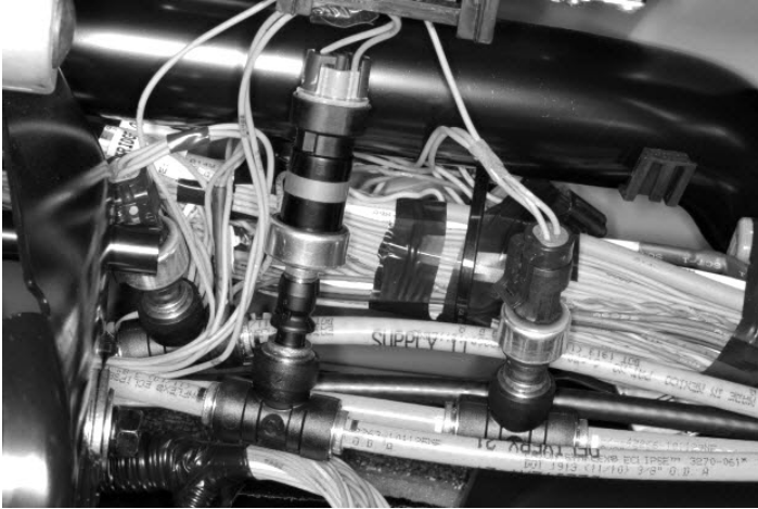
Figure 2 Pressure Switch: Modified Installation
