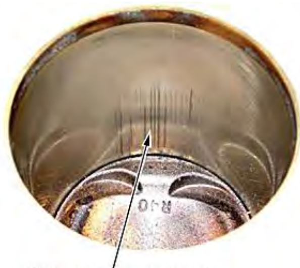
Light scratches are not abnormal. Ensure a fingernail or pencil "catches" on the scratches before replacing the block.
