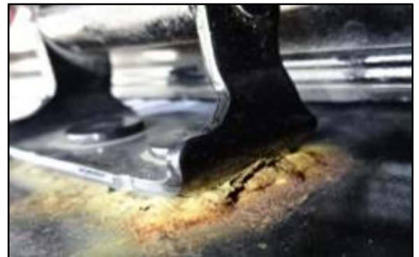
Figure 2. Defined Red Rust
