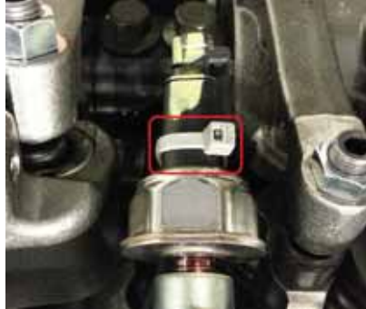
Cable tie location
