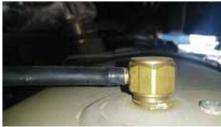
Fuel tank connection
