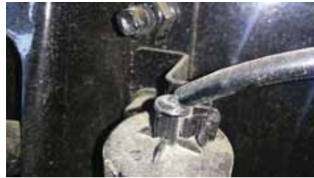
Filter housing connection
