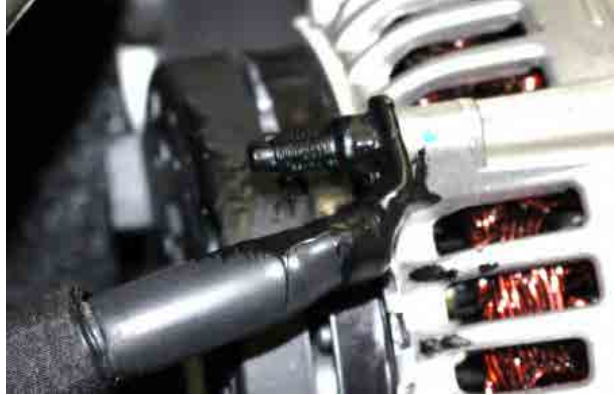
FIGURE 79: GROUND CONNECTION ON THE ALTERNATOR
