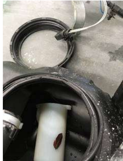
Figure 2. Filter element housing loose inside tank.
