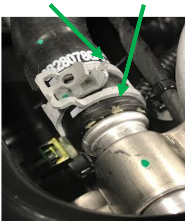
Clamp Pin Visible / No Gap To Hose
