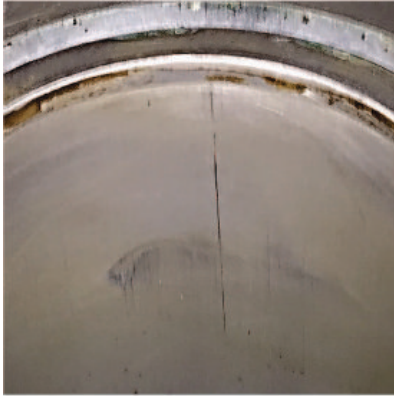
Examples of bore discoloration
