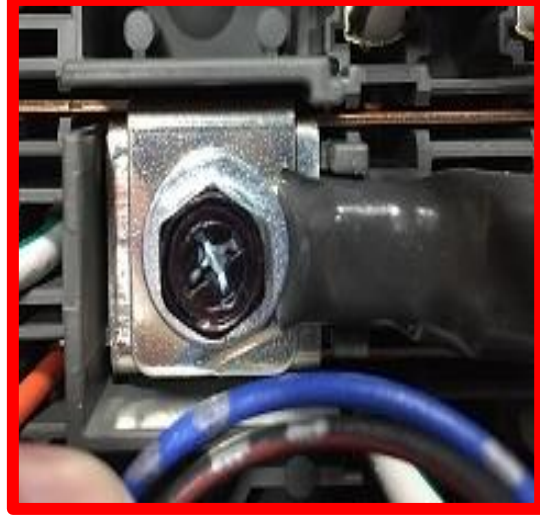
Figure 12 – Not OK Condition
