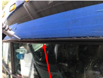
Excess adhesive coming out of fence
