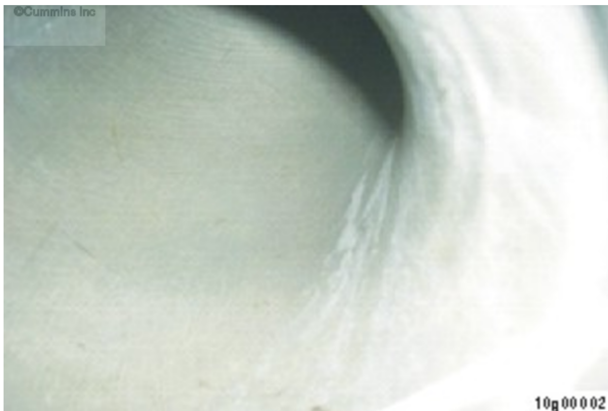
Figure 1, Air intake piping with flux deposits
