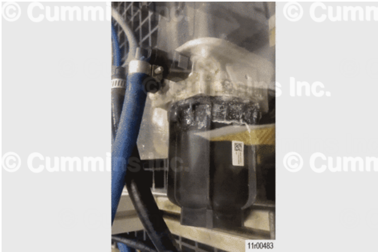
Figure 2, Signs of External DEF Leak Present on Aftertreatment Diesel Exhaust Fluid Dosing Unit.
