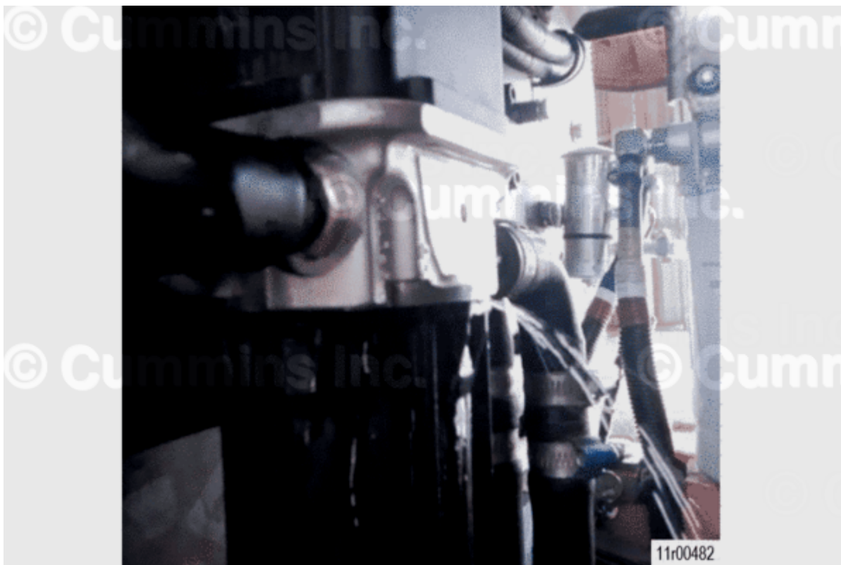
Figure 1, Leak between Aftertreatment Diesel Exhaust Fluid Dosing Unit and Filter Housing.
