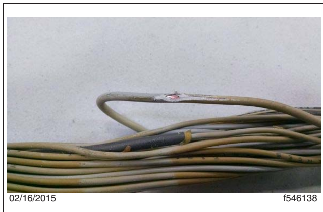
Fig. 1, Worn Insulation, Major
