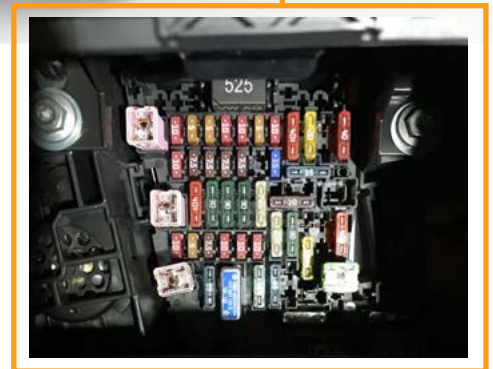
Relay and Fuse Holder SC at the Bottom Left of the Instrument Panel
