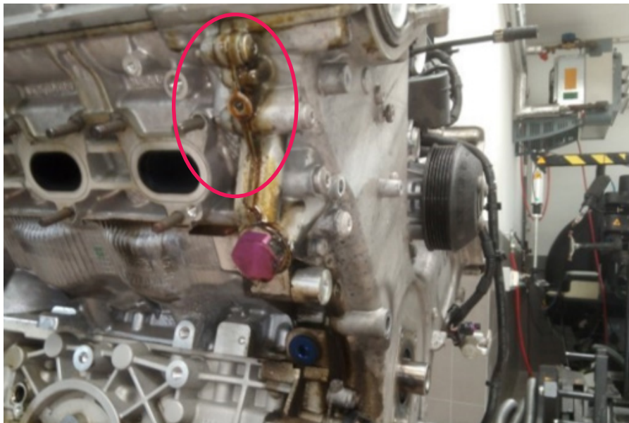
A picture of the location and source of oil leak with engine clearly removed is required
