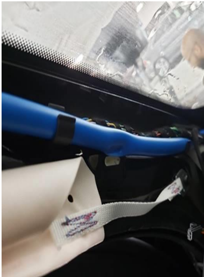
Figure 2. Sunroof drain hose pinched by pillar trim.
