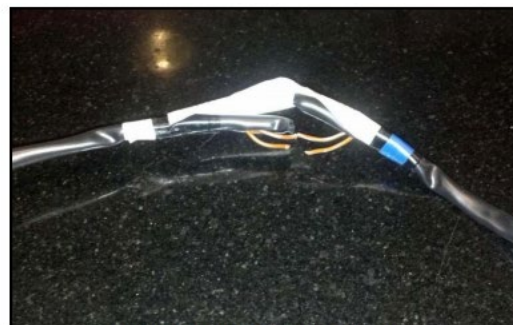
Close-up View of Damaged Harness
