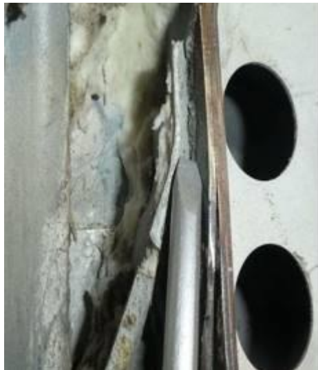
Figure 16. Incorrect engagement of the chisel end.
