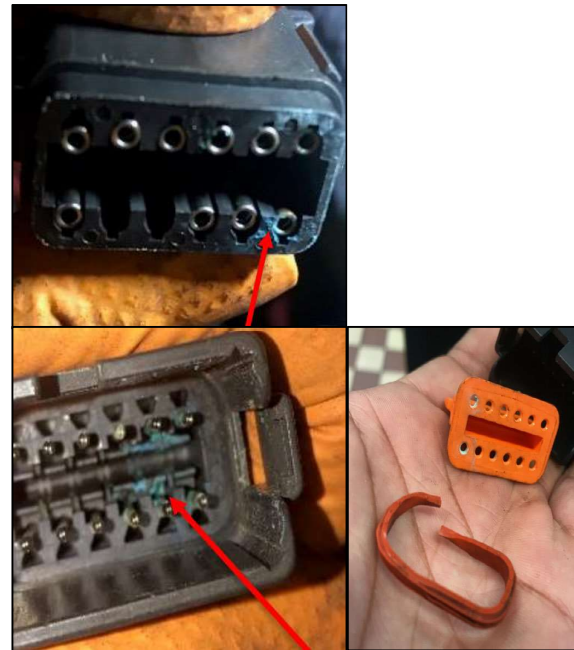
Figure 7 – Examples of Corrosion and Damaged Mating Seal
