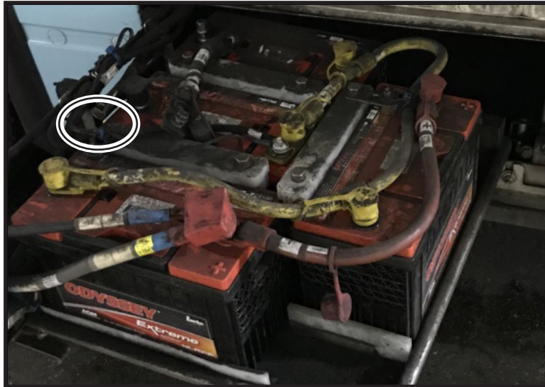
Figure 4 - Ground Cable Disconnected and Isolated
