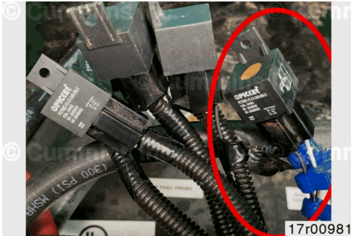
Figure 3, Harness relay circled in red
