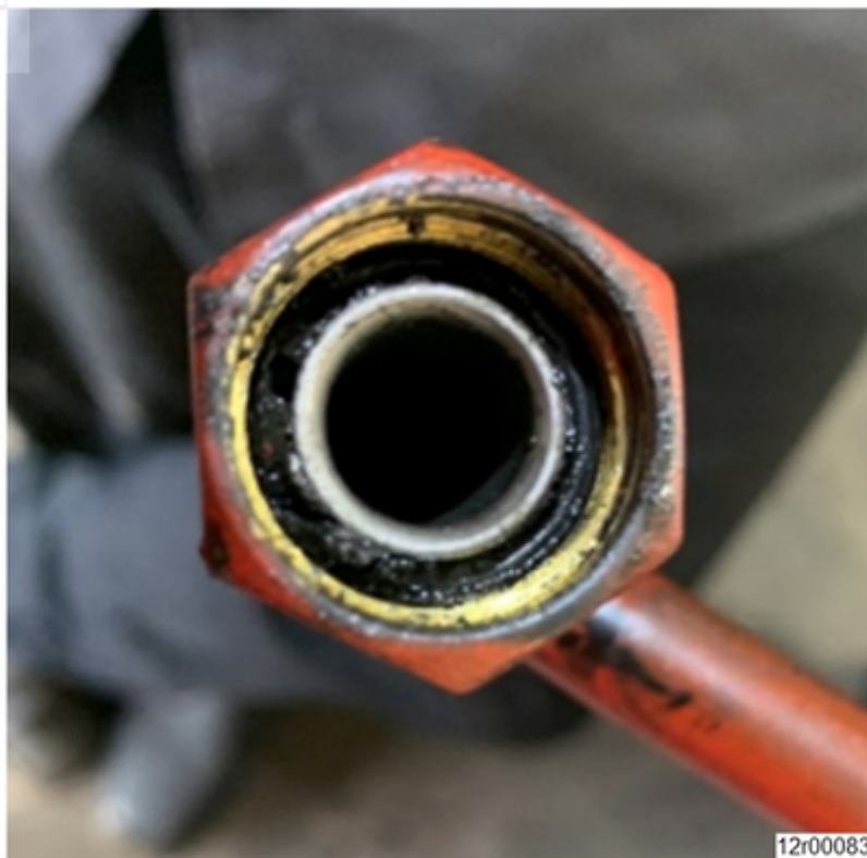
Figure 1, Example of Deteriorated Grommet.
