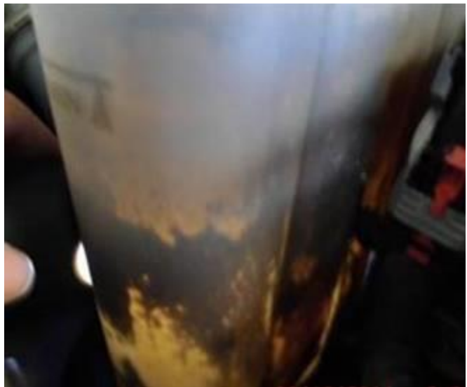
Figure 12. Discolored coolant expansion tank.
