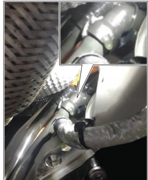
Friction welded joint for ATF cooling line faulty
