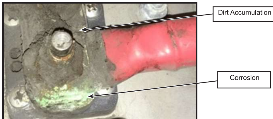
Figure 9 - Junction Bus Bar and Power Cable Lug
