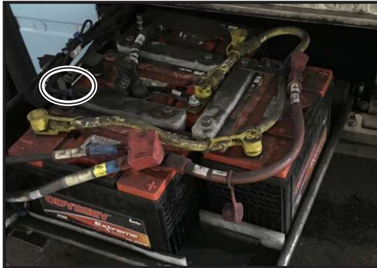
Figure 4 - Ground Cable Disconnected and Isolated
