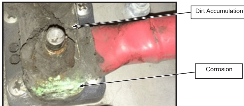
Figure 9 - Junction Bus Bar and Power Cable Lug
