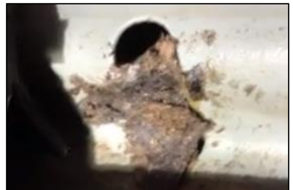
Figure 5. Example of Debris on Drain Hole
