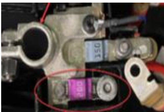
Figure 1. Fuse S164 circled in red.
