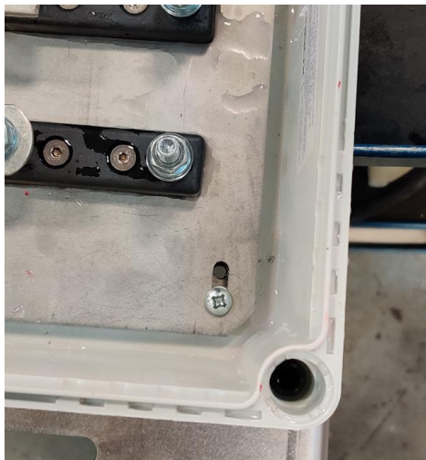
Figure 1: Drilled hole in the bottom corner of the fuse box allowing water draining.
