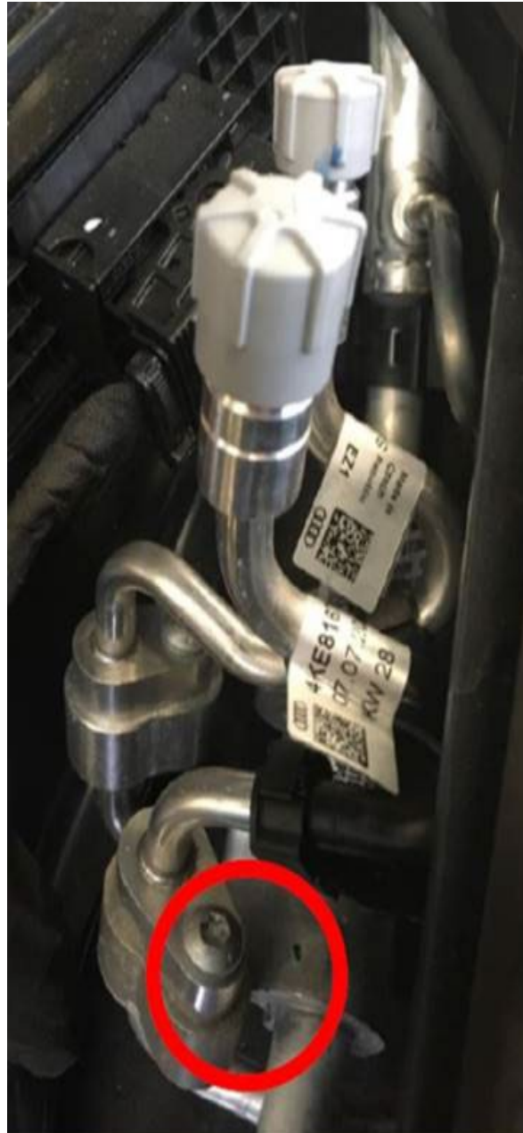
Figure 2. The refrigerant lines are making contact.
