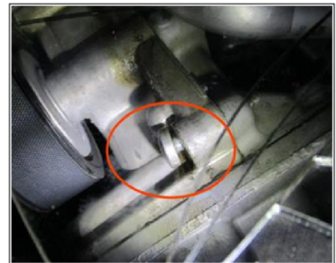
Sample illustration: Loose/broken screw in the chain housing cover
