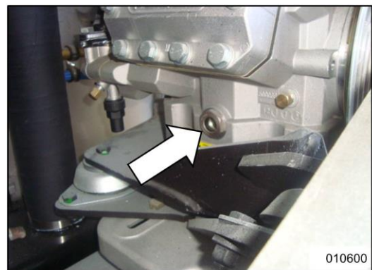
Figure 2: Oil level sight glass on Eberspächer/Bitzer refrigerant compressor.
