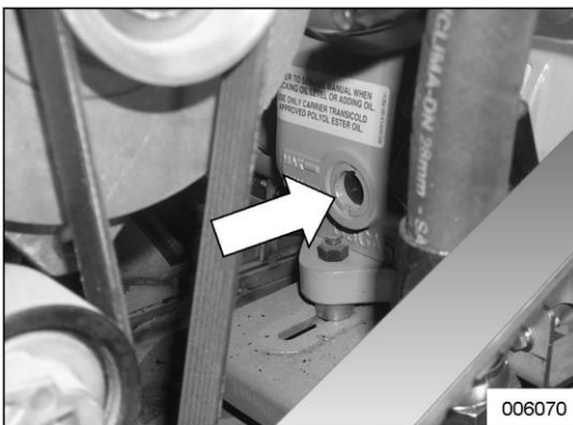
Figure 1: Oil level sight glass on Carrier O5G refrigerant compressor.
