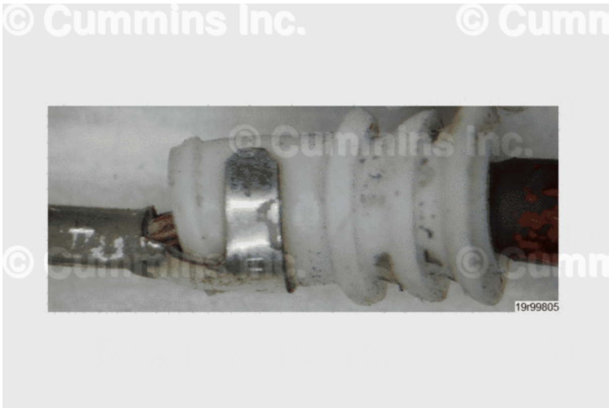
Figure 3, Copper Wire Strands Within the Ground Terminal Showing Signs of Corrosion.
