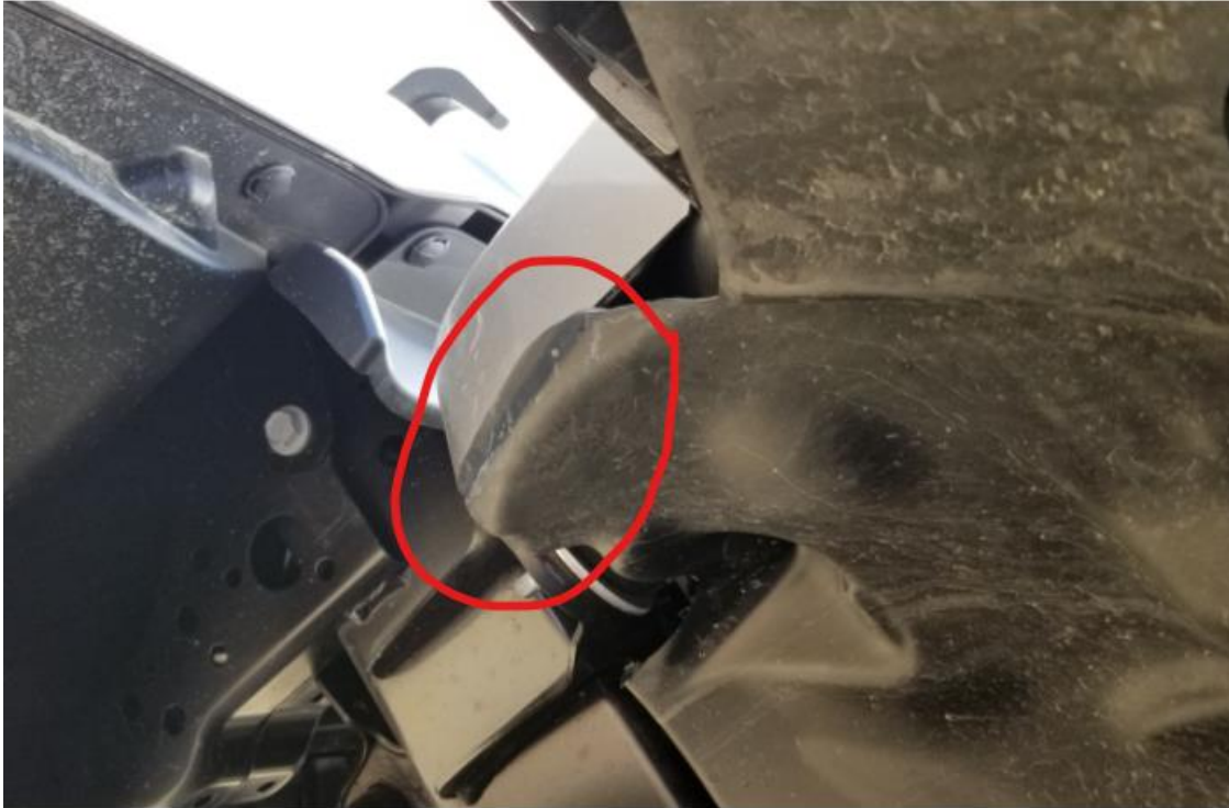
Example of the liner not tucked behind the grille.
