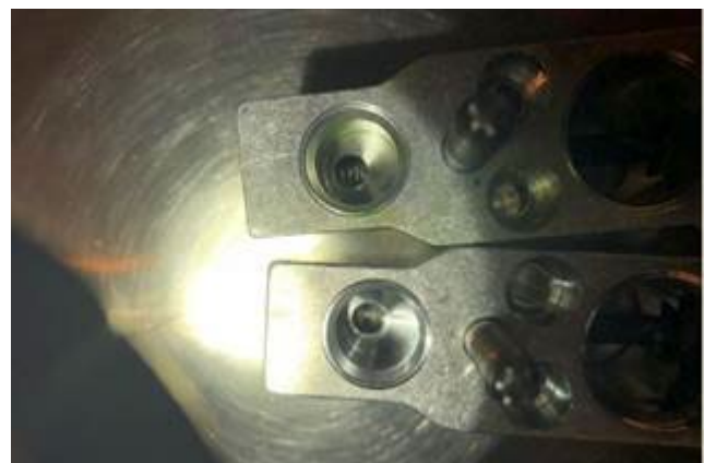
Figure 4. Leak at expansion valve connection evidenced by residue from the contrast agent.
