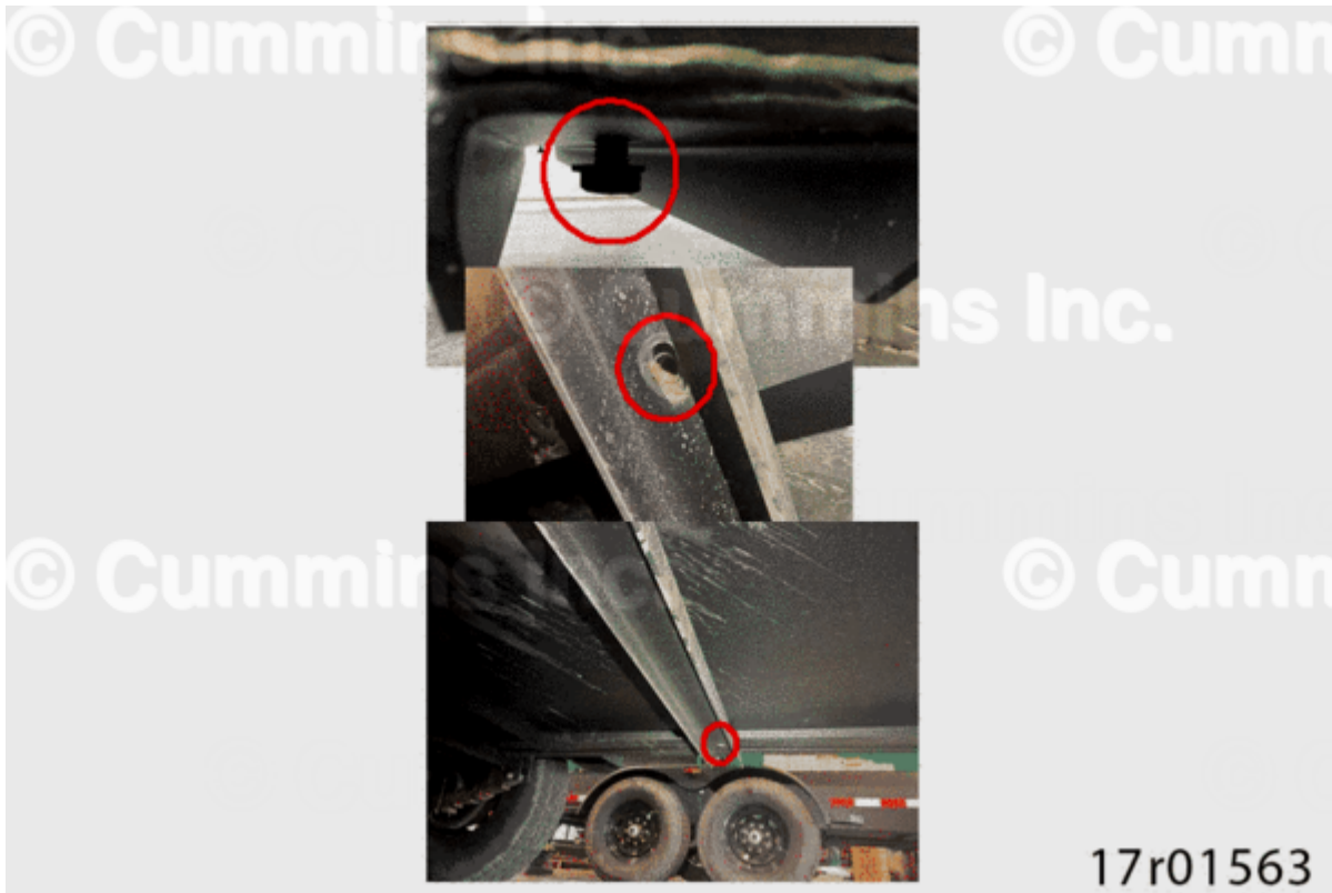
Figure 1: Loose and missing trailer bolts
