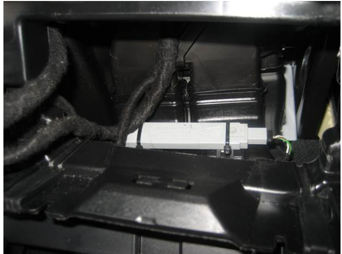
Figure 8. Aerial 1 mounted on HVAC ducting.
