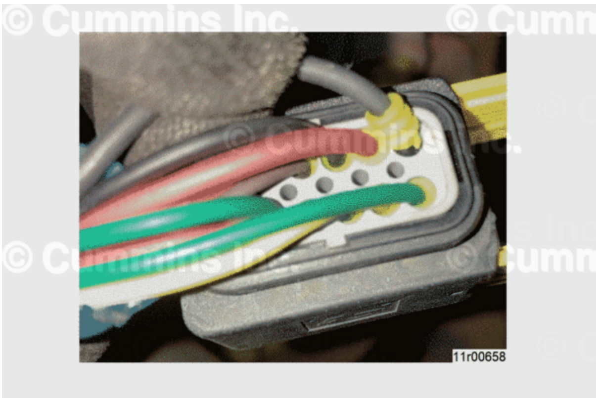
Figure 2, Loose Wire at Back of OEM Wiring Connector to Aftertreatment DEF Dosing Unit.
