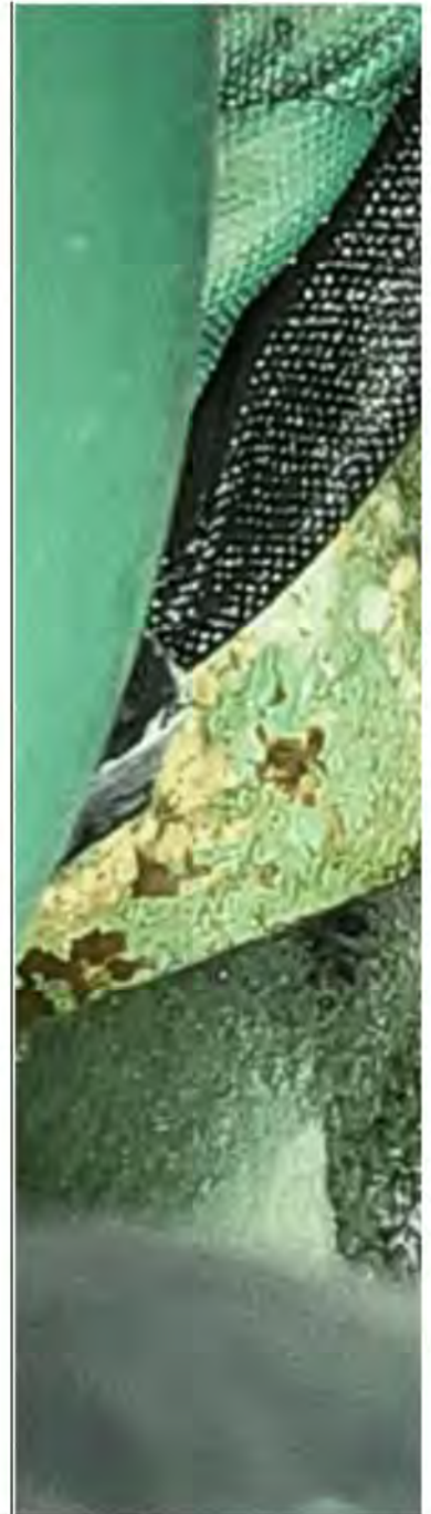
Oil actively leaking
