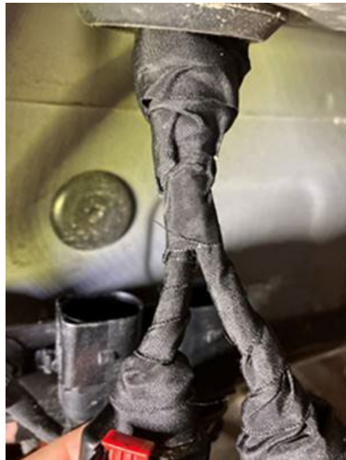
Figure 6: Harness fully repaired.
