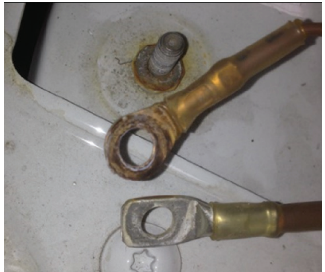
Figure 2 - Example of corrosion on ground point
