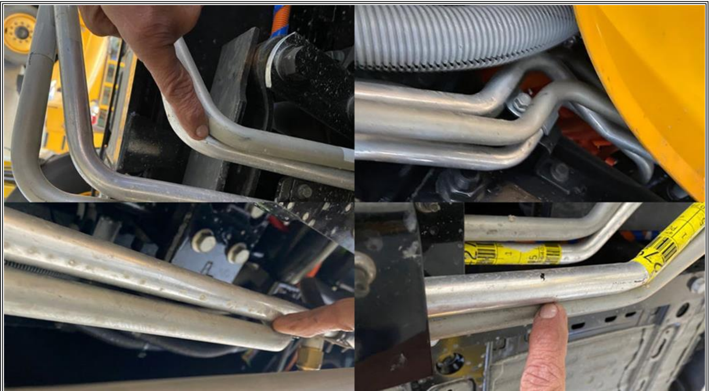
Figure 1: Examples of coolant pipe contact
