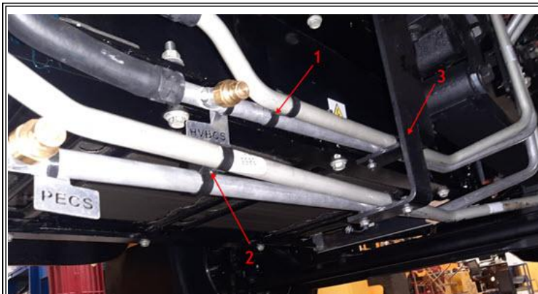
Figure 4: Installed Cable Straps Location 1 & 2
