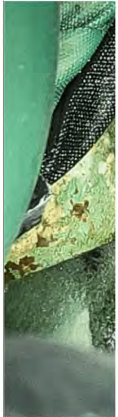
Oil actively leaking
